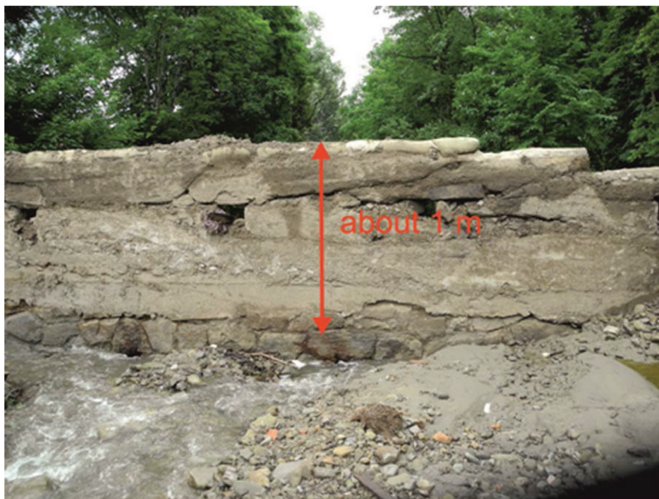
Figure 1. Heightened part of the dam, as seen while emptying of the reservoir
