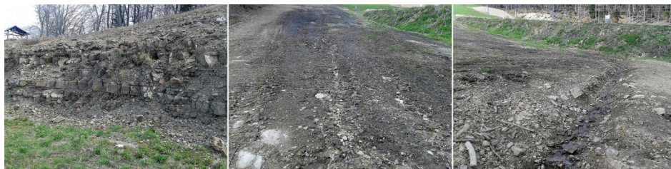
Figure 3. An example of the scope of engineering works and anti-erosion measures performed in the ski slopes areas. Photo by J.Gołąb
