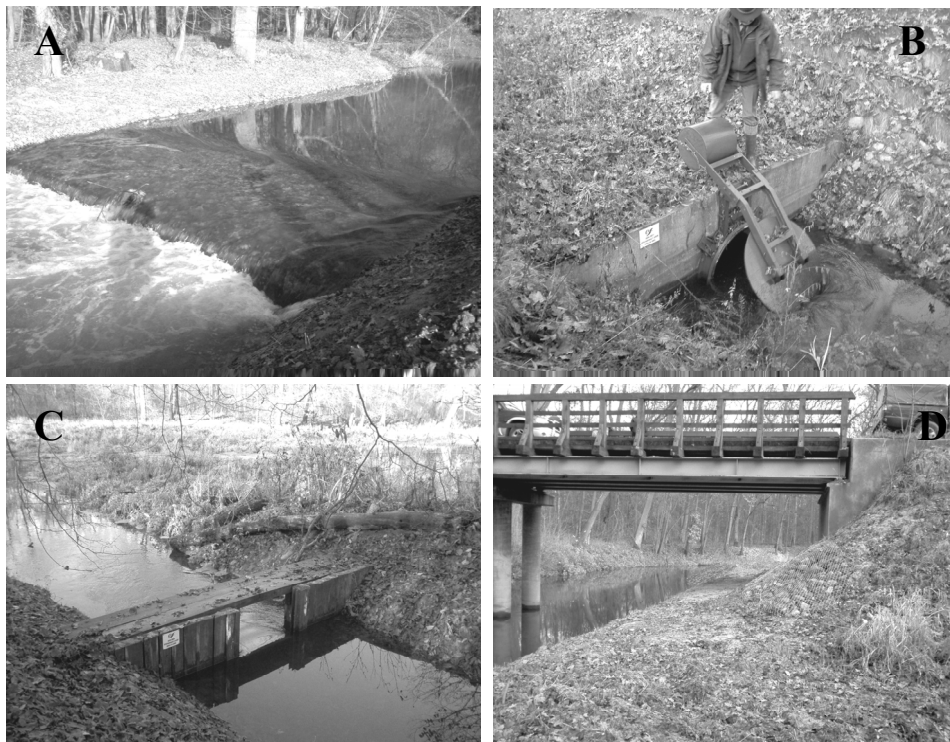
Figure 4. A damming sill (A), a culvert with a flap check valve (B), a log stop gate (C), a bridge on the Lutynia River (D)
