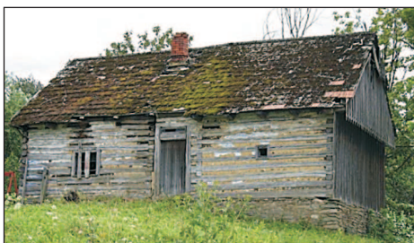
Phot. 70. An abandoned and dilapidated building of the end of the 19th century (photo: P. Herbut)
