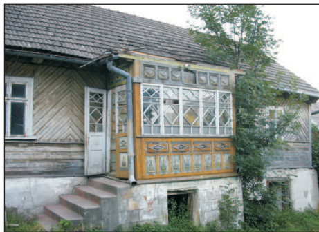
Phot. 68. An abandoned and dilapidated house of the beginning of the 20th century (photo: W. Bieda)
