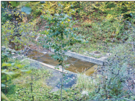
Phot. 33. Surface water intake in Lipnik (photo: G. Kaczor)
