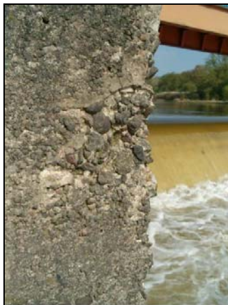
Rysunek 2. Jaz Opatowice. Odslonięte grube kruszywo na przyczółku (stan 2006 r.) Figure 2. Opatowice weir. Washed out concrete with uncovered coarse aggregate on the abutment of the weir (state in 2006)
