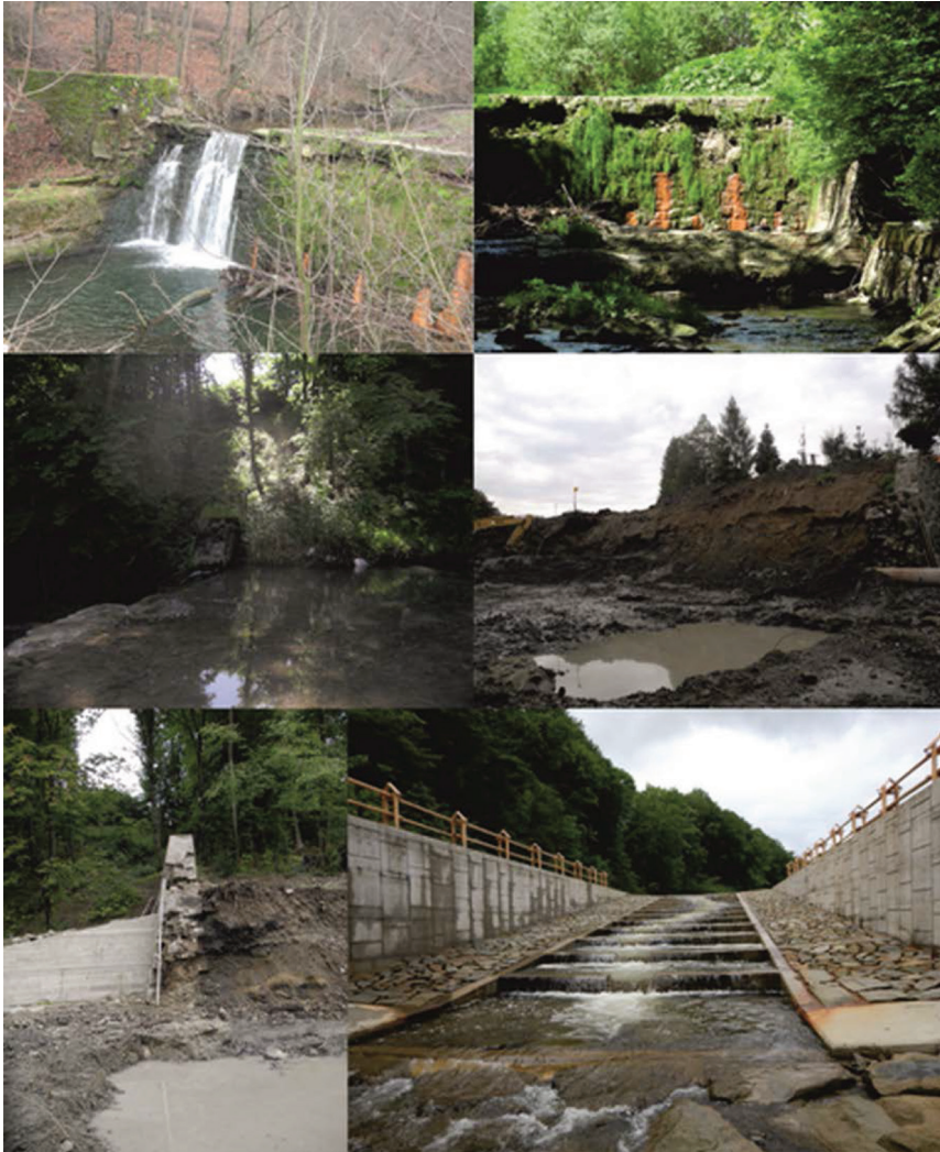
Figure 3. From the top clockwise: The dam seen from downstream – year 2012 and 2015; view upstream; reservoir after dam and deposit removal; cascade of basins in place of the main dam body; old dam remains, reservoir before the work commenced
