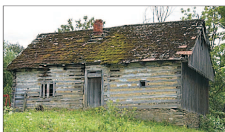
Phot. 70. An abandoned and dilapidated building of the end of the 19th century (photo: P. Herbut)
