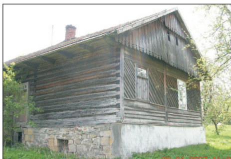
Phot. 50. A house covered with clapboards with an underpinning plastered only from the front: the gable is separated from the wall with a double overhang finished up with a decorative detail (photo: W. Bieda)
